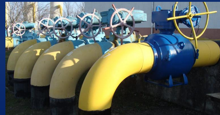
Pipe elbows of gas transportation system
