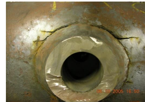
In-service failure of a branched connection
