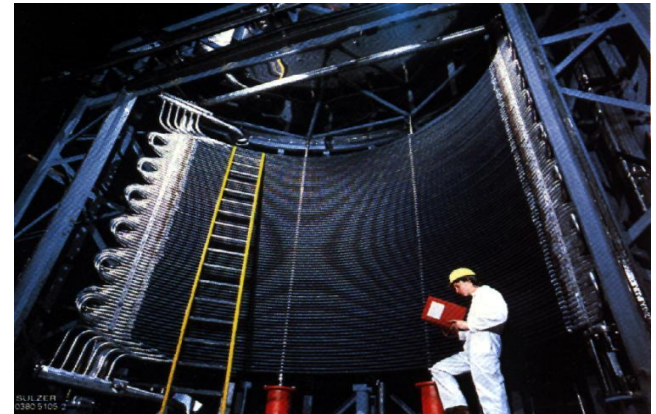
Tube-bundle solar receiver
